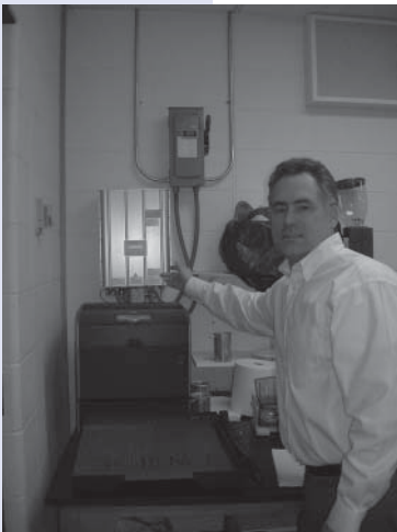
Pictured above is Science ID, Jim Sullivan pointing out the inside equipment that runs the solar panel.
